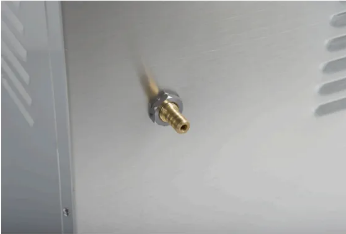
Automatic cold-air exhaust.
